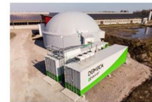
Biodegradation® -biogas plant Wennström Ilpo's farm
