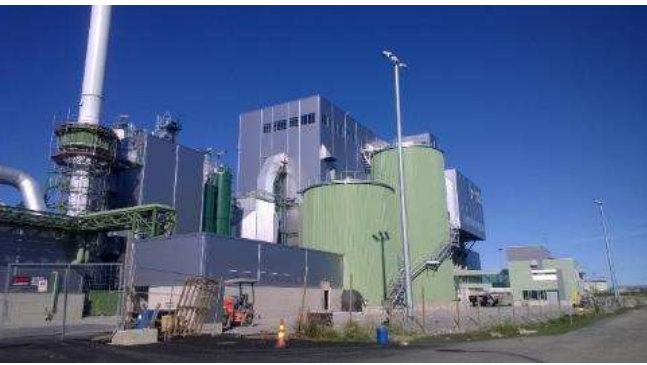
COMMERCIAL POWER PLANT IN TARASTENJÄRVI (100 Gwh), Tammervoima Oy, Prefabrication And Implementation Phase.
