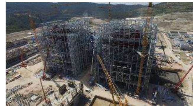
SOMA KOLIN BOILER (CFB) FACILITY, TURKEY FOSTER WHEELER 2 x 255 MWe
